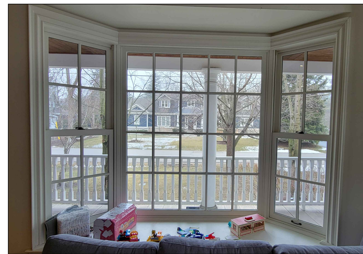
LOCATION IMAGE REFERENCE FOR WINDOW PANES ONLY CASING TO BE AS DETAILED IN DRAWING
